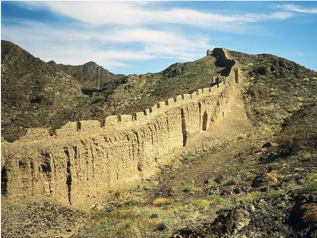
View of a part of the Bahla town-wall in its ruinous condition in the early 1990s. Photo: Georg Popp.
